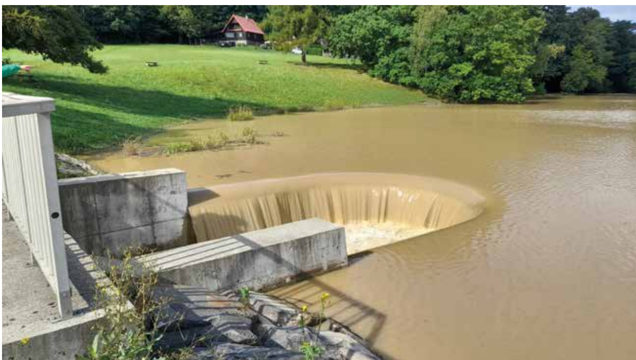
Spillway of the Kletná small water reservoir on the Kletenský Brook in operation on 29 August 2022
