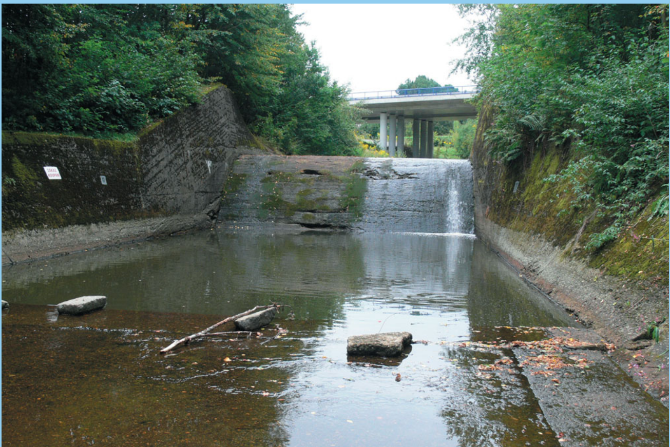
Step 11 before the repairs
