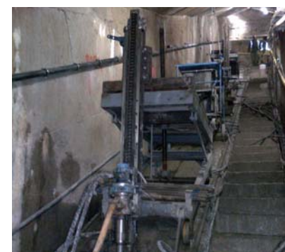
Reservoir Šance – The additional left-hand side sealing and joining / the injecting of the drilling
